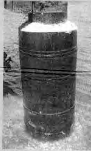
Severe Damage Piling Encapsulation
