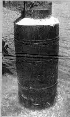
Severe Damage Piling Encapsulation
