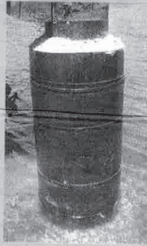
Severe Damage Piling Encapsulation
